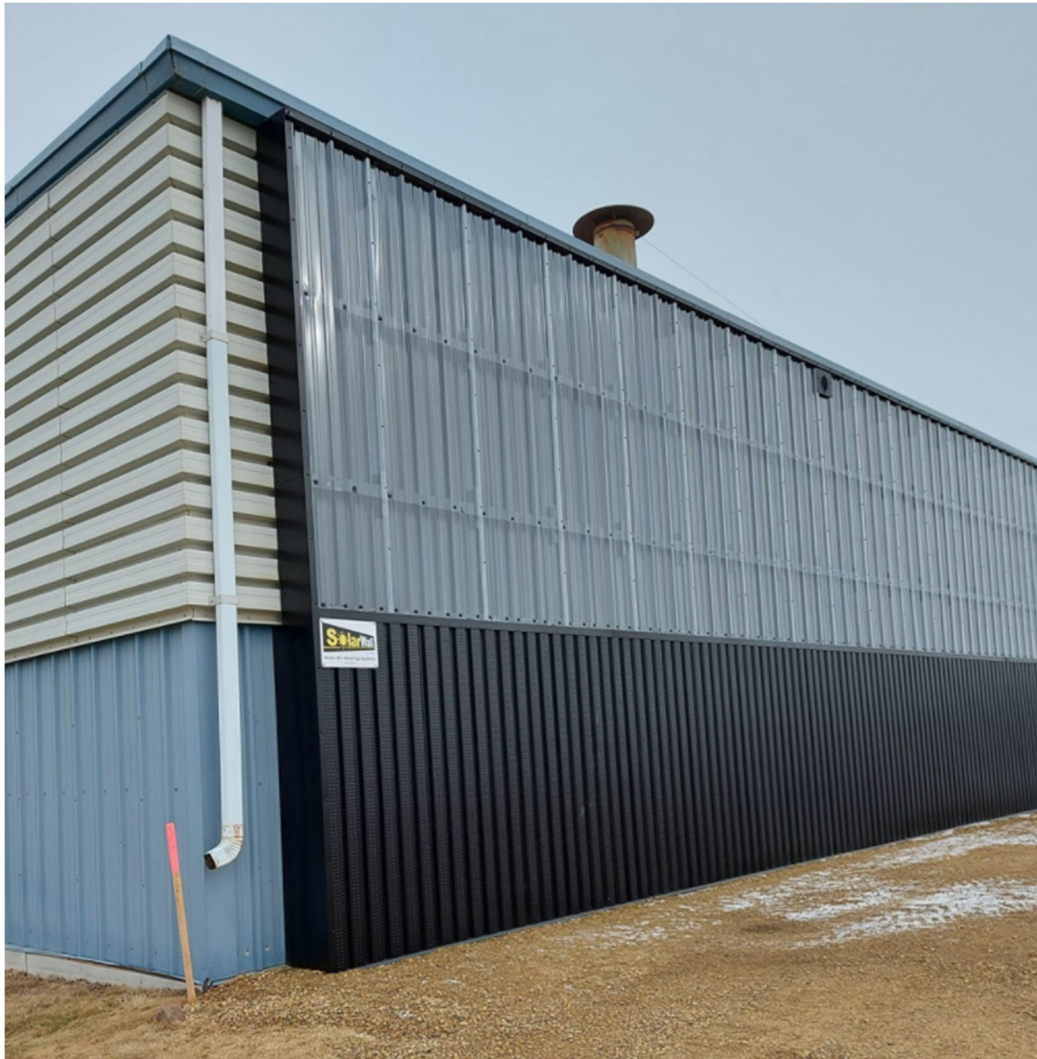
The 2-stage SolarWall® transpired solar collector on the south wall of the HKRWSC water treatment plant.
